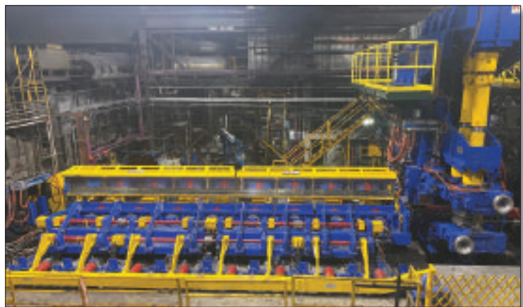
Fig 1 Insulated roller table and rolling stand typical configuration
