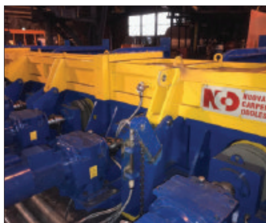
Fig 2 Insulated roller table
